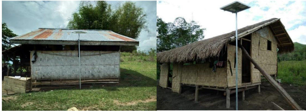
Sample Roof-side Pole mounted installations
